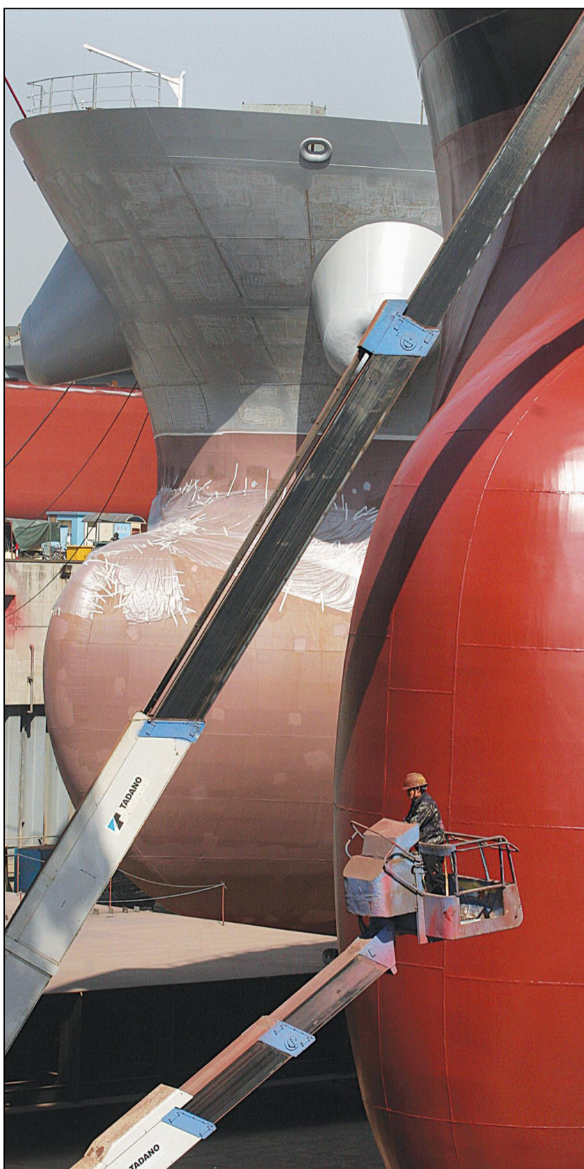
A capesize bulk carrier under construction in Shanghai: the market collapse and freeze on bank lending has hit cashflow at Chinese and South Korean yards. Bloomberg
